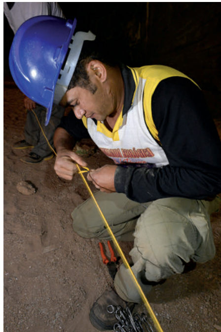
Photo 12 to 15 – Examples of poly-cord trail installation processes in the dark part of Janelão Cave
