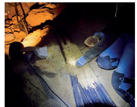
Figure 3: Covering a large cable run with mud paste and loose fill. Photo by Evan Hubbard.
