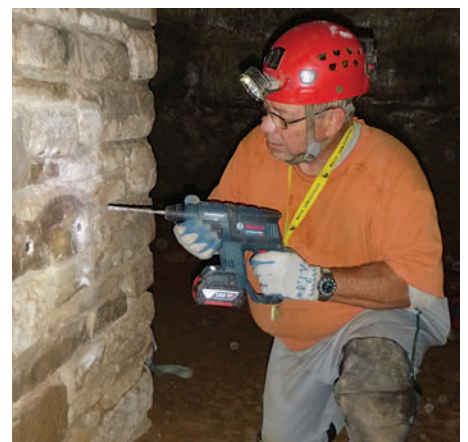
Resto caver and former camp director Bill Copeland uses a drill to remove lead anchors from a stone wall in Mammoth Cave.
